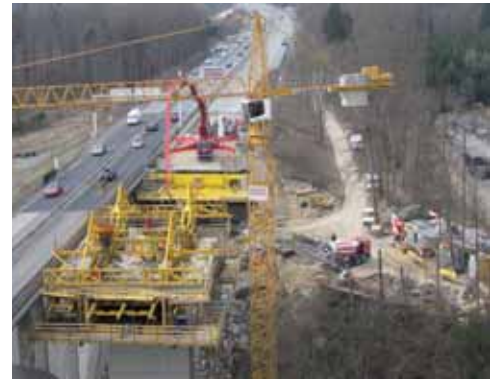
Mega construction site. Renovation work on the River Traun bridge on the A1 at Steyrermühl, Austria.
